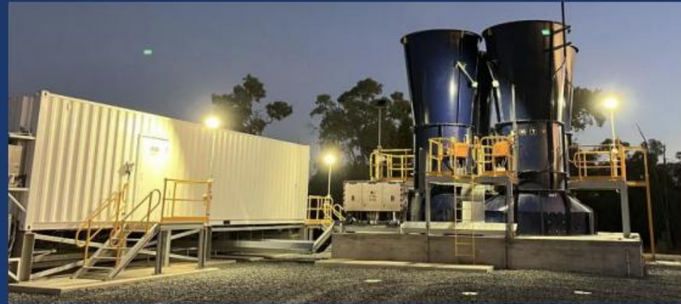
Photo: Surface ventilation fans
