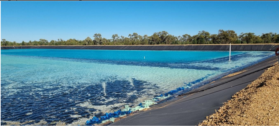
Photograph 11 – Water Management Dam
