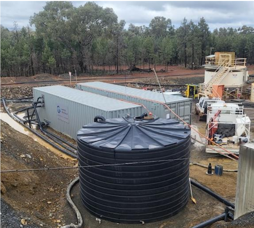
Figure 3: Hired water treatment plant commissioned and now operating.
