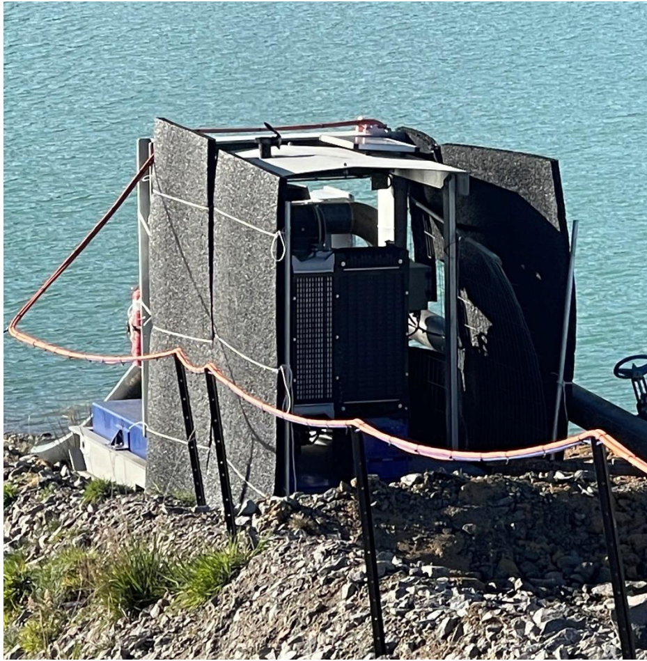
Photograph 3 - TSF Pump Noise Attenuation
