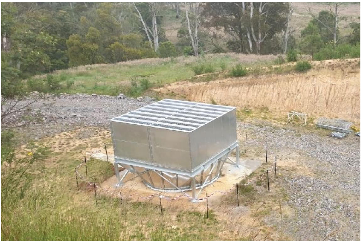
Photograph 2 - Ventilation Fan Silencer
