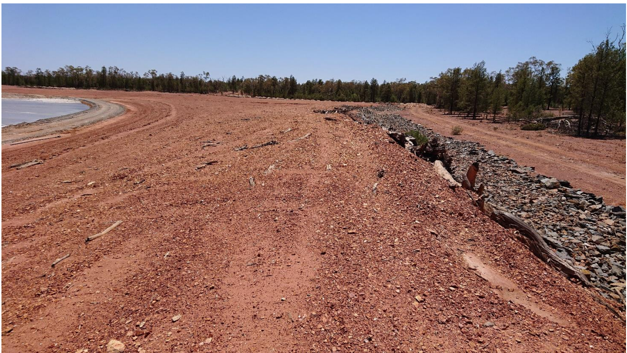
Photo # 5 - TSF Clean Water Diversion
