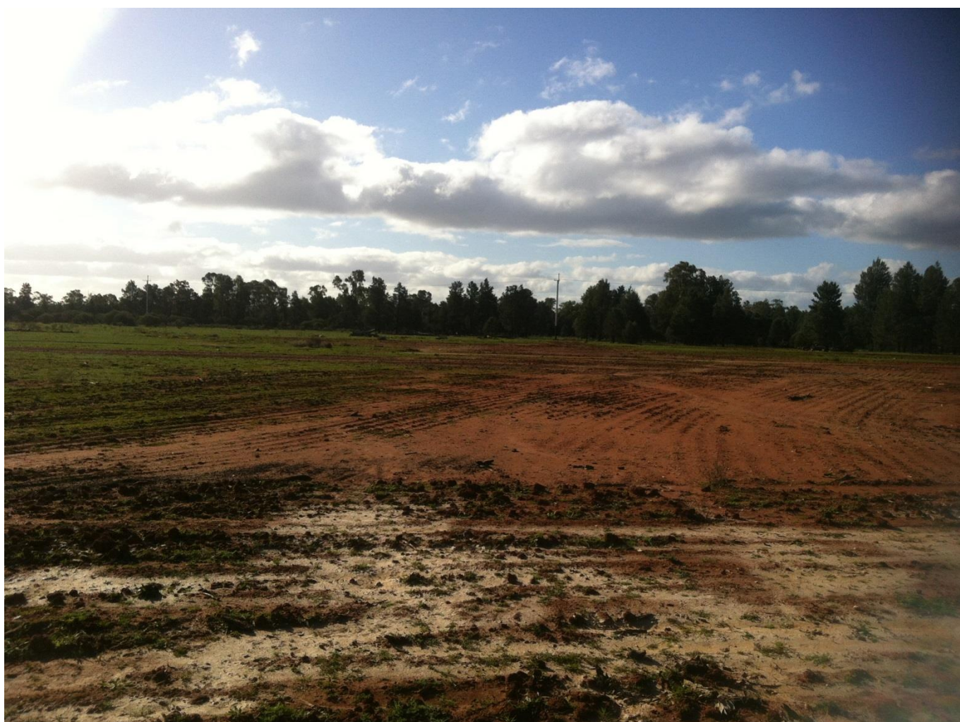
Figure 5.2.1 A photo looking north of the old laydown yard that was decommissioned in this reporting period.
